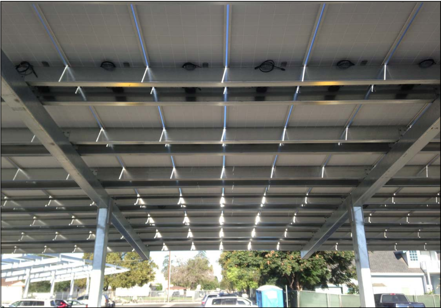
Carport solar panel system was installed offsetting 82% of campus daily demands.
